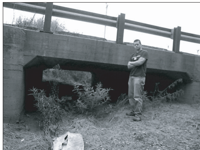
Figure 8. Example of a large concrete culvert located within tenth mile section 25.0. Dimension are roughly 4 x 20 x 25 ft. During dry seasons culvert are utilized as underpasses by animals, as indicated by deer and raccoon tracks. A large female deer carcass was located on the left side of the road's shoulder (out of view). Another small deer carcass was discovered in the bush to the left.
