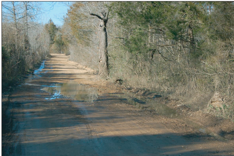
Figure 7. A location where a cross drain is needed to reduce sediment production.
