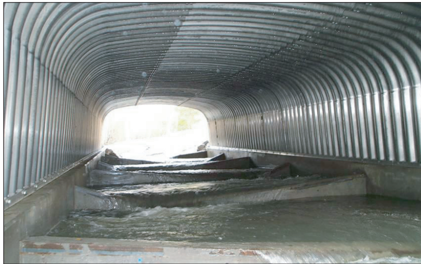
Figure 3. Vertical walls used to provide resting pools for fish may trap terrestrial animals. A horizontal shelf along the edge of the culvert is a possible retrofit to allow terrestrial animals dry walking space. Photo from Fish Xing.
