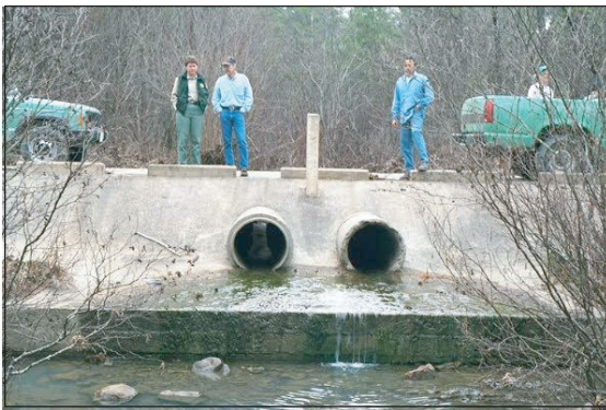
Figure 4. Vented low-water ford fish barrier.
