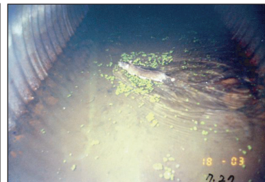
Figure 7. Inundated circular culvert.
