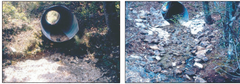
Figure 1. Rusted out pipe with drop. Figure 2. Gouted pipe and riprap ramp.
