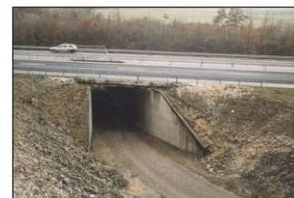
Fig. 3. 2 nd generation of fauna passages. Underpass at the A5.
