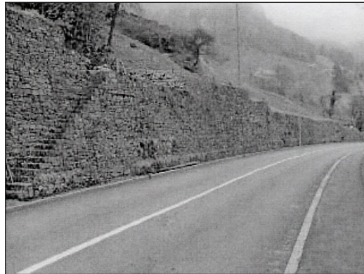
Figure 11. This retaining wall built with gabions can be climbed by various animals, reducing the strong barrier effect such structures normally exert. The crevices of the coarse material provide habitat to small animals and plants.
