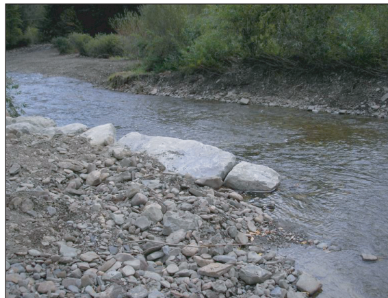
Figure 12. One of the rock vanes built on the north bank of Canasawacta Creek. The photo was taken looking downstream.
