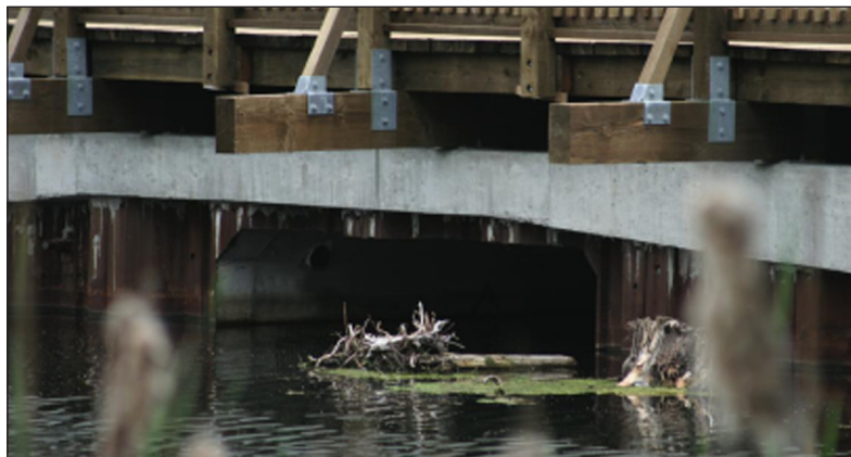
Figure 5. Wet culvert at McKenzie Wetland for fish, waterfowl, reptile and amphibian passage.
