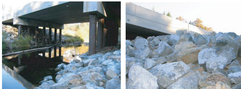
Figure 5. Bridge replaced in 2007 with excellent shape and size to allow passage for all terrestrial species present in the area, but rendered impermeable for many terrestrials due to the large boulder armament. This type of abutment protection is very common in current bridge replacements. Photos S. Jacobson.
