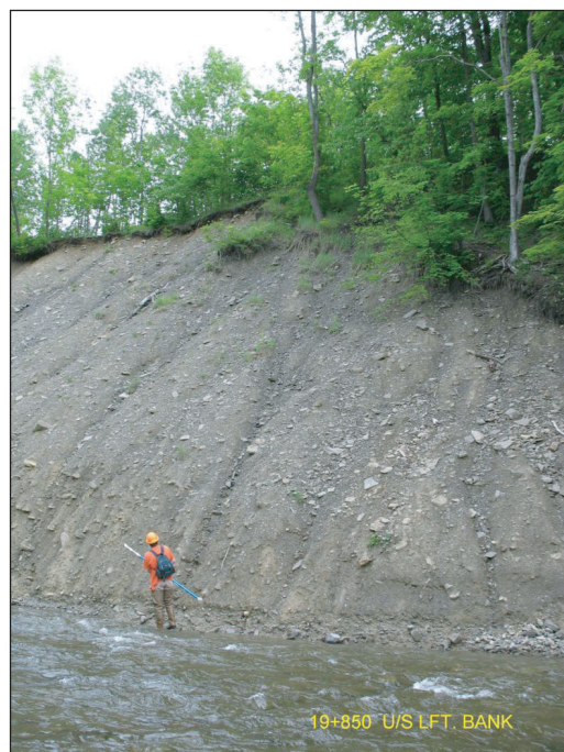
Figure 5. Eroding south bank of Canasawacta Creek just upstream of the Moon Hill Road bridge. Material is continually sloughing off into the creek.
