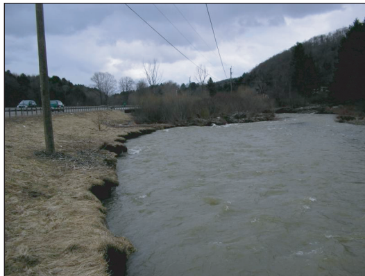
Figure 9. Looking downstream just above of the Chan Aldridge bridge in March 2006. Notice that the utility pole is several feet from the creek. It had already been moved once so that it was not engulfed by the stream.
