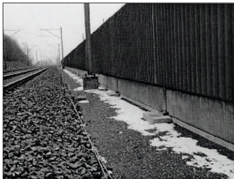
Figure 8. Noise barrier along a railroad line.
