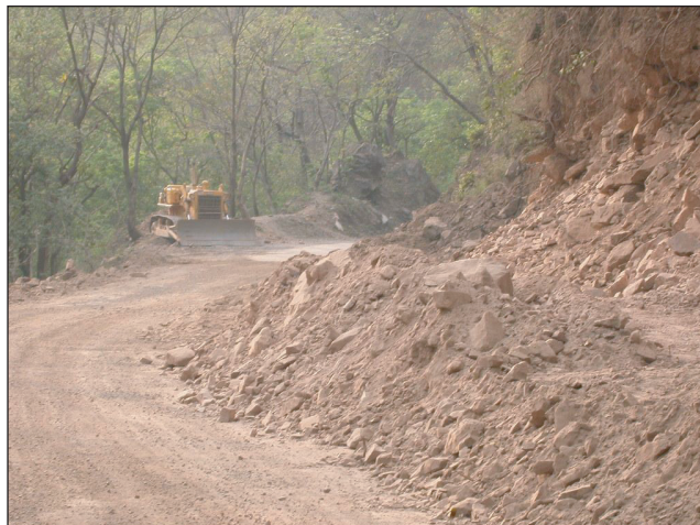
Figure 2. Landslides caused by uncontrolled blasting during road construction and widening along the upper Ganges.
