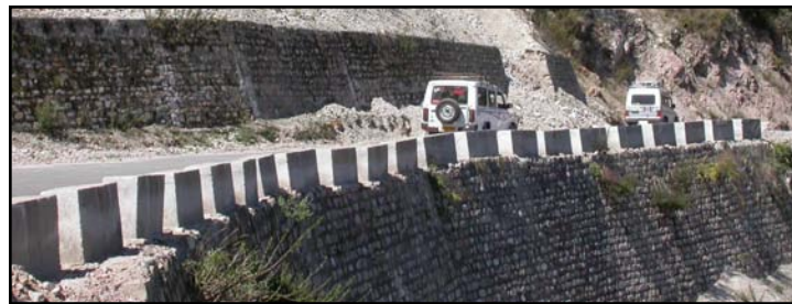
Figure 6. Early failure of toe wall due to heavy precipitation during monsoon (July-August) on NH-58.
