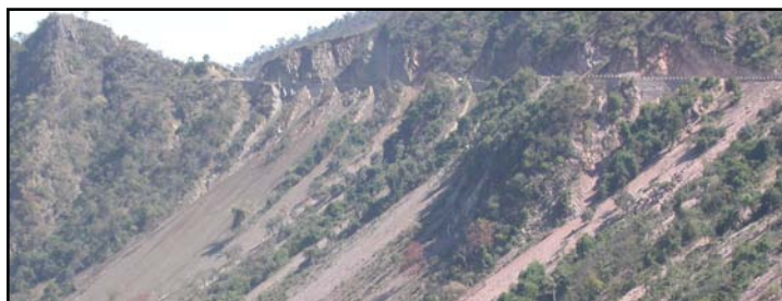
Figure 1. Disposal of cut material downhill into the Alaknanda River caused by the widening activities on NH-58.
